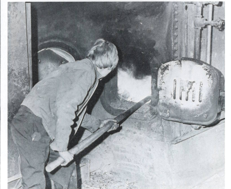
John works at keeping everyone warm by keeping the boiler hot
