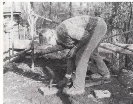
Rusty Pulling Nails
