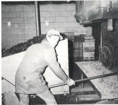
Dan fires the boiler to keep us warm.
