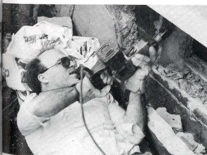
Mr. Hess cuts a hole to install a new air-conditioner at the san.
