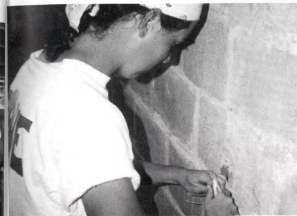
Nicole strips some wires in preparation for hooking up a switch box.
