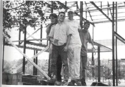
Jerod, Andrew, Scott, and Ben stand on the steel pieces used to construct the Quachita Hills Academy building they are working on.
