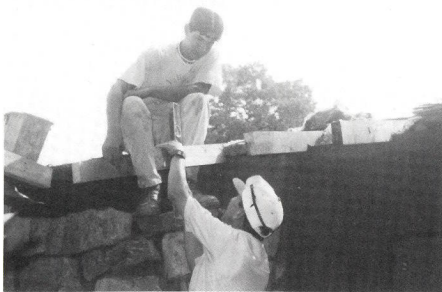
Mr. Zamora and Jeremy work together to fix the boys' dorm roof.
