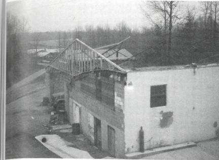
The construction crew begins to build the roof trusses for the shop extension.
