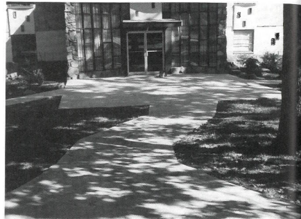
We worked long and hard on our new sidewalk in front of our Administration Building.
