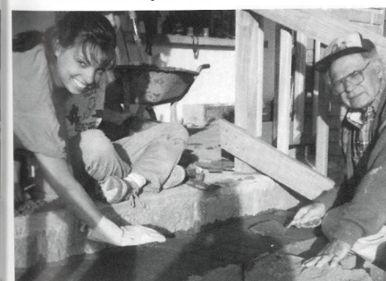
Mr. Bob and Janelle lay blocks for the steps on their project.
