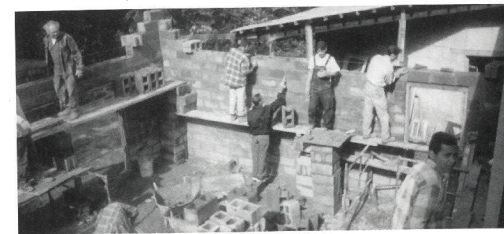
The Layman's Foundation workbee accomplished much on the new school building addition.
