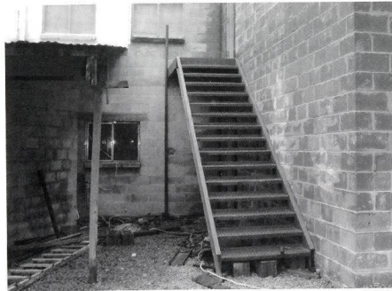
Progress has been made on the addition to the main classroom building. Mr. Bob and his student helpers built this fire escape.
