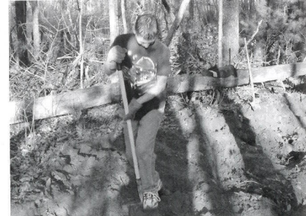
Norbert helps fill in a pipeline ditch for the new sewer extension.
